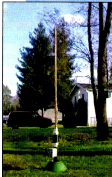
Nice Sticks! The www.sstran.com site shows construction details for a high-efficiency Part 15 compliant AM antenna system with loading coil and transmitter mounted at the base ( www.sstran.com )
