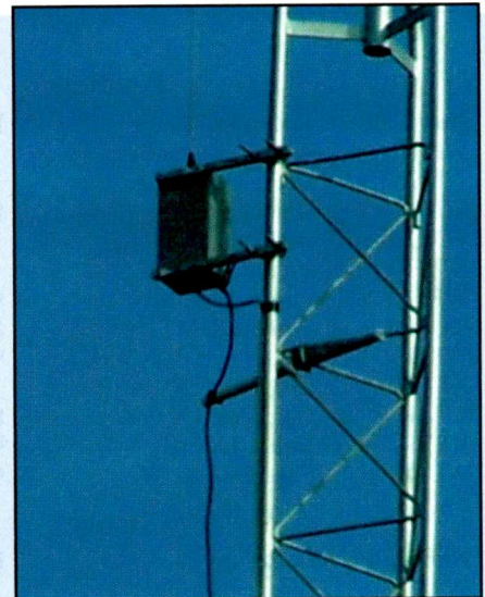
The 1690 Adventist Radio transmitter box is shown here with whip antenna mounted on a tower.
